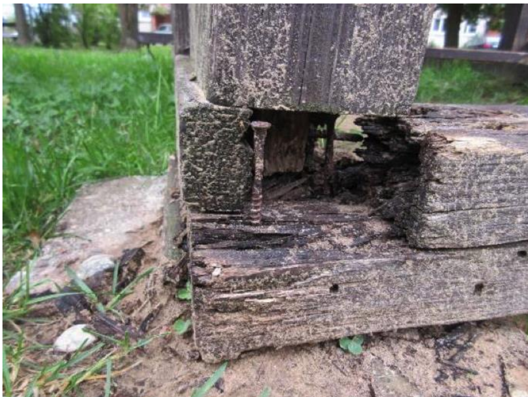
Photograph 7 Example of damage that may lead to collapsing/breaking down of the equipment
