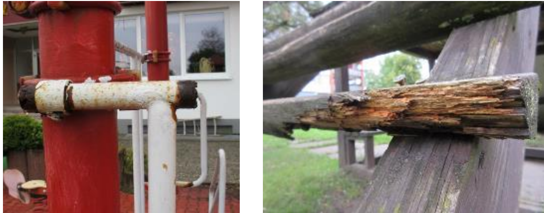
Photograph 6: Lack of structural integrity non-compliance
